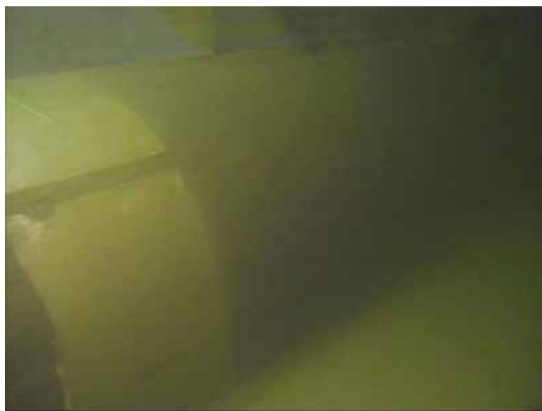
Figure 11-7. Anode around the pipeline on the seabed seabed to protect from external corrosion. ©Nord Stream
