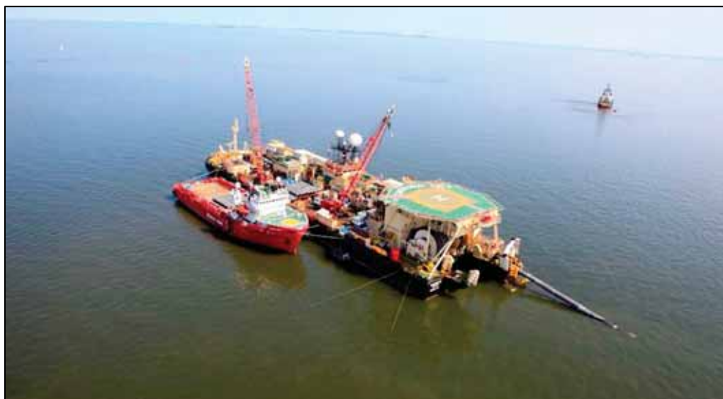
Figure 6-22 Typical shallow water lay barge (with anchor tug and pipe transportation vessel).
