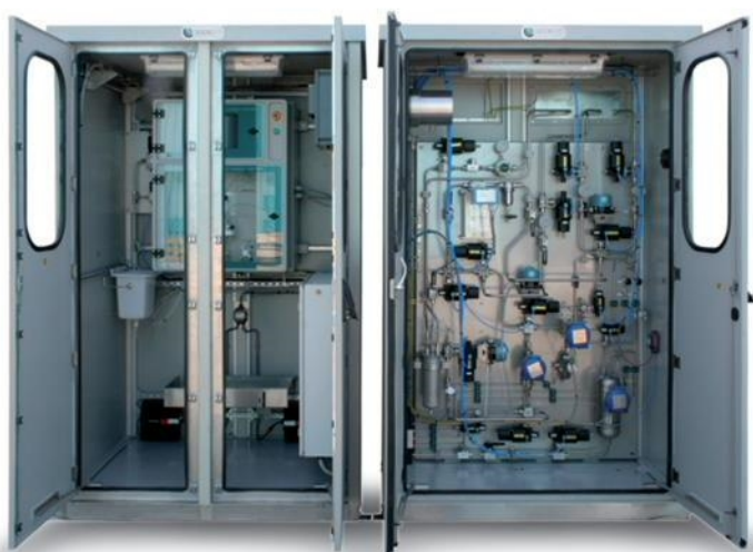
Analyzer shelter with integrated sample preconditioning system
